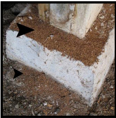
The black arrows indicate termite droppings, which look like piles of mud or dirt.
