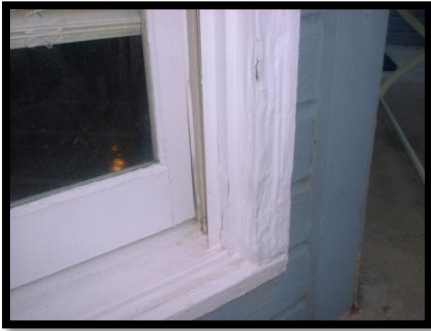
The bubbling/rippling paint along this window frame is a clear indicator of a termite problem.
